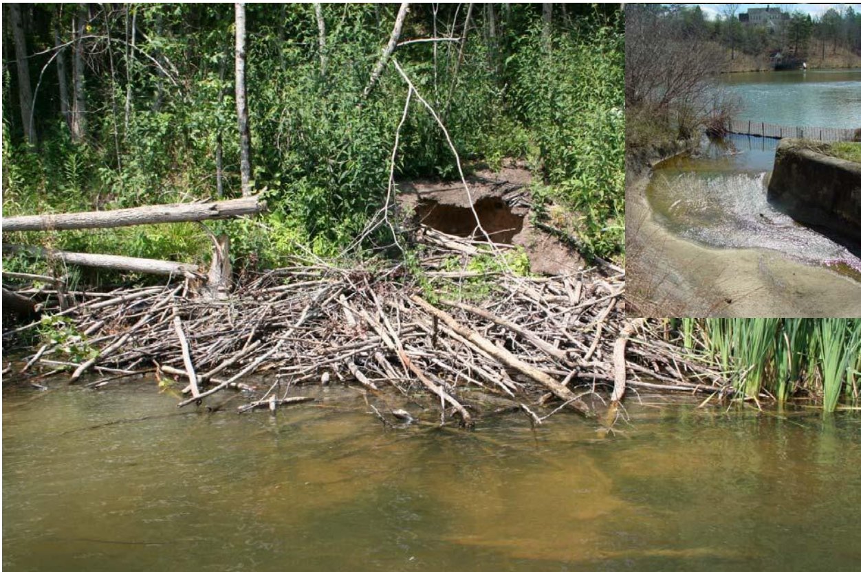
Beavers and muskrats can bore in to the side of the dam and weaken its structure. Emergency spillways should be lined with concrete if they receive heavy flow (inset).
